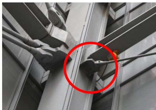
FIGURE 2- 'Dog-leg' penetrating building envelope
